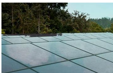
65 kw solar power plant.
