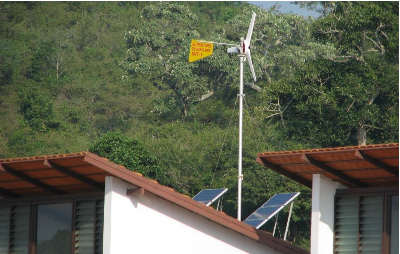
Combined wind and solar generation at Dhole's Den.
