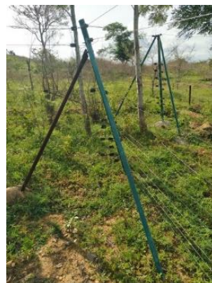
Solar powered fencing.
