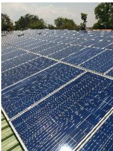
Solar thermal supplies all the resort's hot water.
