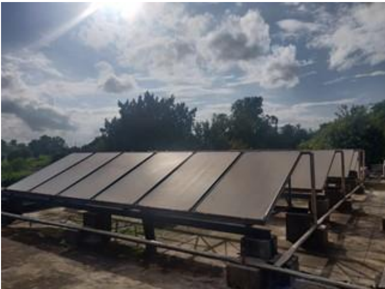
90 kw rooftop solar plant.
