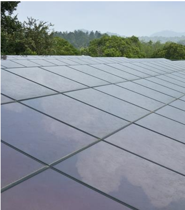
65 kw solar power plant.
