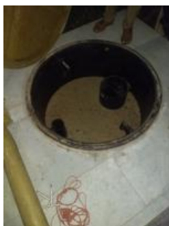
Grease trap behind the kitchen.
