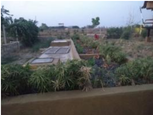
Phytorid water treatment....
